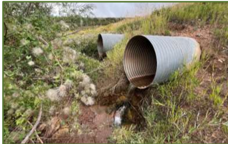
Perforated pipes at southern pond
