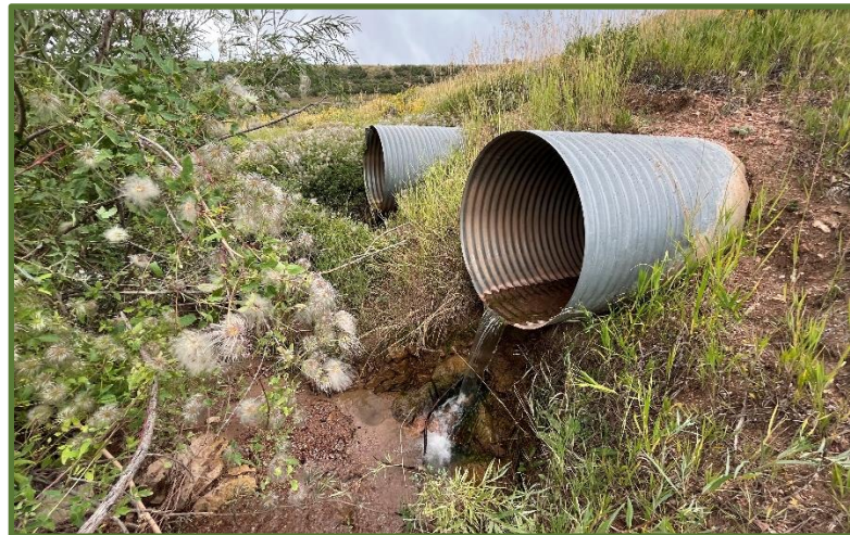
Perforated pipes at southern pond
