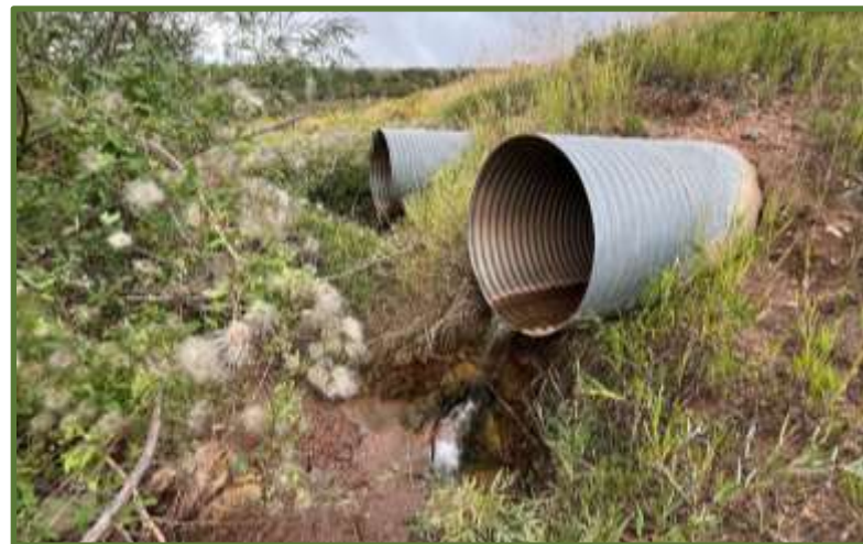
Perforated pipes at southern pond
