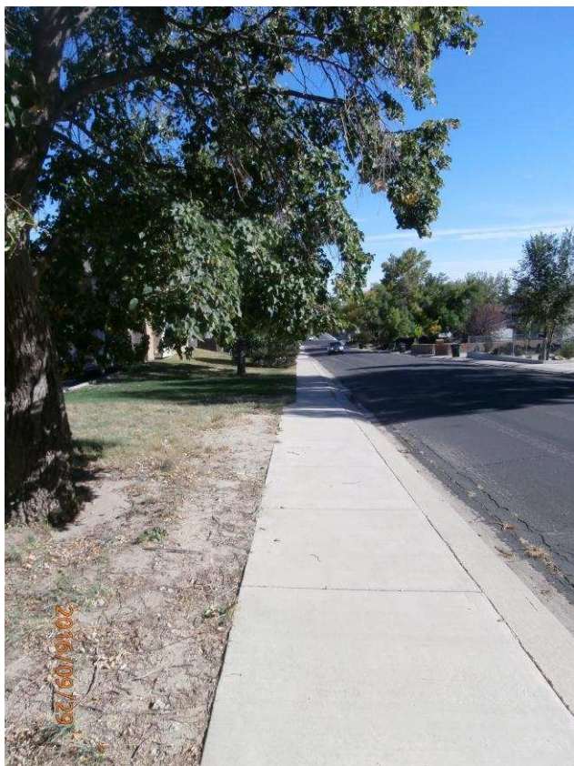
Tree branches hang within 80" of the sidewalk
