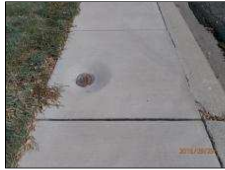
Water main access is recessed in the sidewalk
