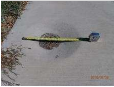
Watermain access recessed in the sidewalk
