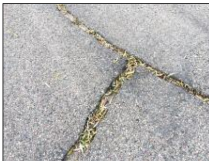
Gaps in the asphalt parking
