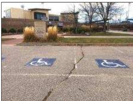
Accessible parking spaces are not compliant
