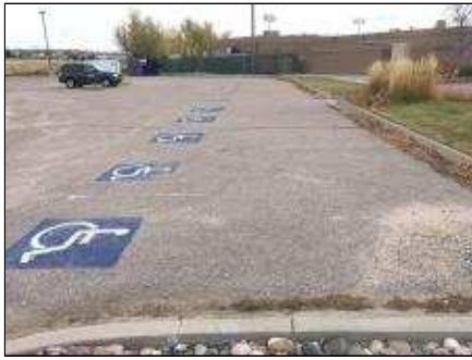
Accessible parking striping is faded
