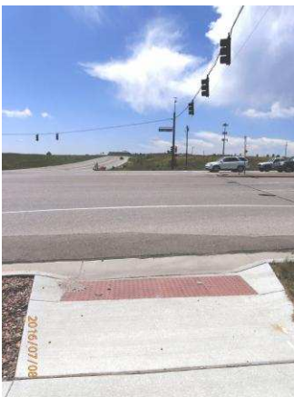
Image of lack of connecting curb ramp
