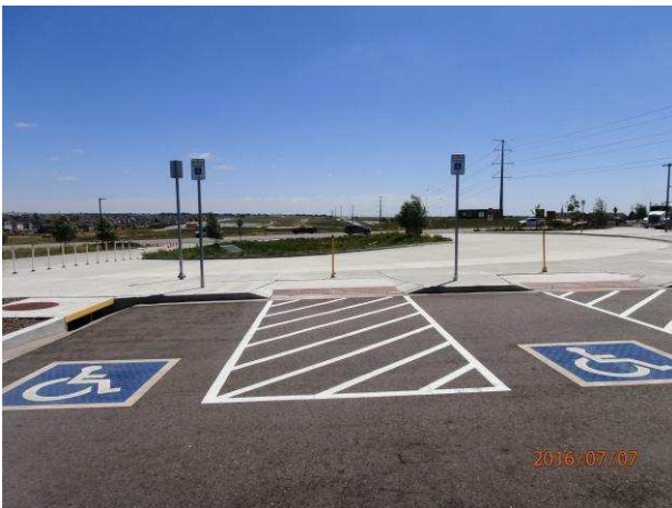
Image of obstructed curb ramp landing
