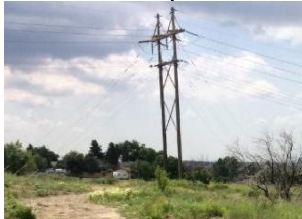
Electric transmission tower and lines will be undergrounded as part of this project.
