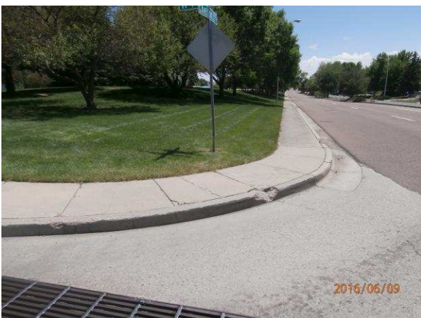
Image of curb head without curb ramp
