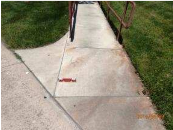
Additional image of noncompliant ramp
