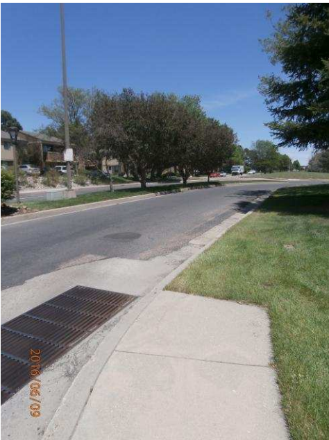
Image of sidewalk abruptly ending
