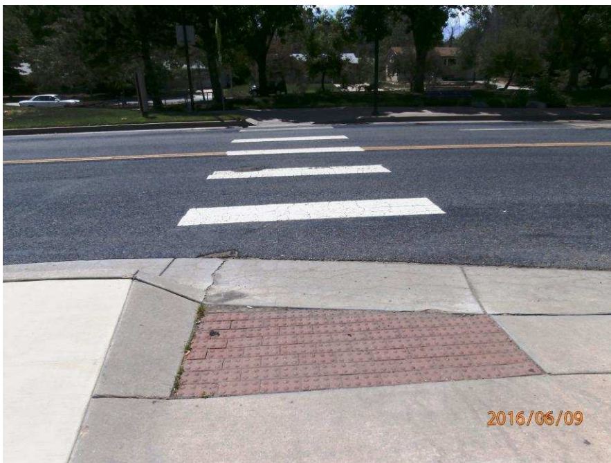
Image of noncompliant curb ramp
