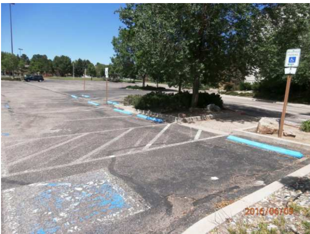
Image of accessible parking spaces without signage
