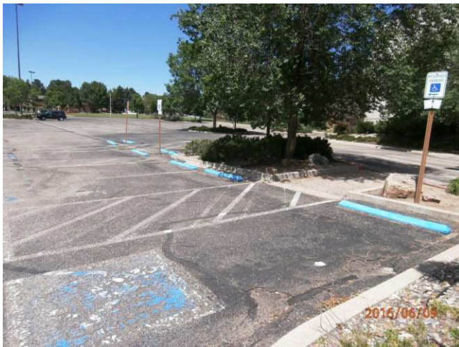
Image of deteriorated pavement in the accessible parking space
