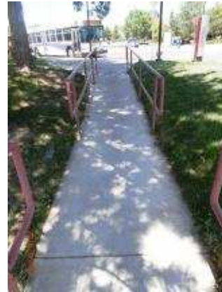
Additional image of noncompliant ramp
