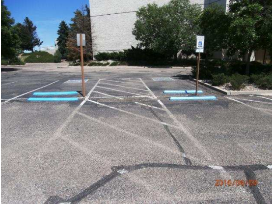
Additional image of faded markings on the parking spaces
