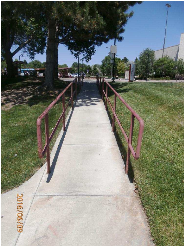
Image of noncompliant ramp
