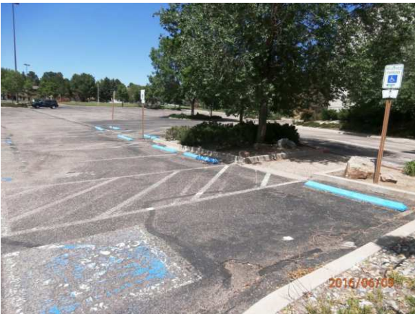
Image of faded van accessible signage
