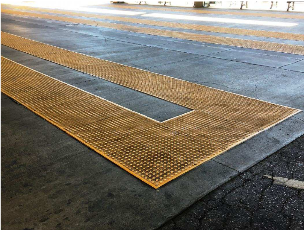
Image of noncompliant dome pathway
