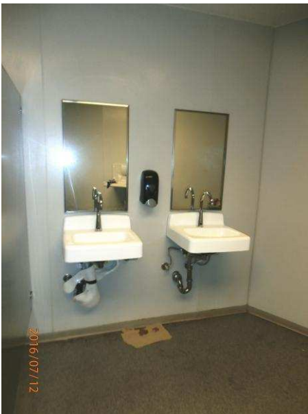
Image of noncompliant lavatory
