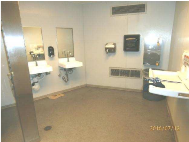
Image of paper towel dispenser mounted too high
