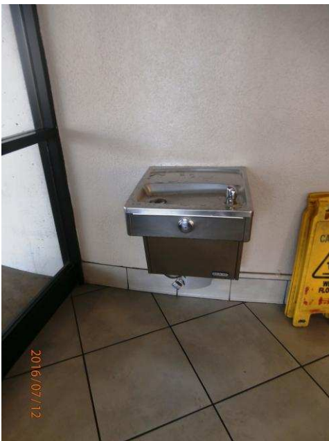
Image of noncompliant drinking fountain
