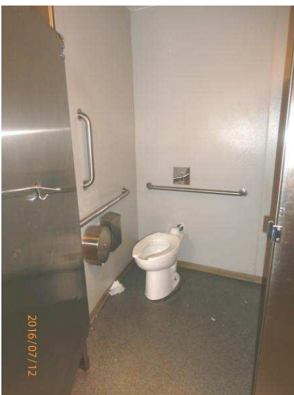
Image of toilet too close to wall
