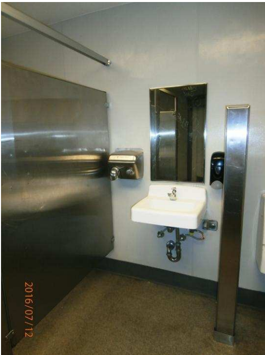
Image of lavatory without pipe insulation
