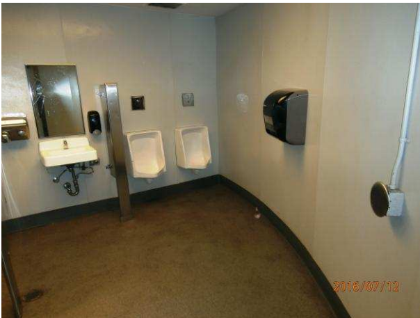
Image of urinals mounted too high
