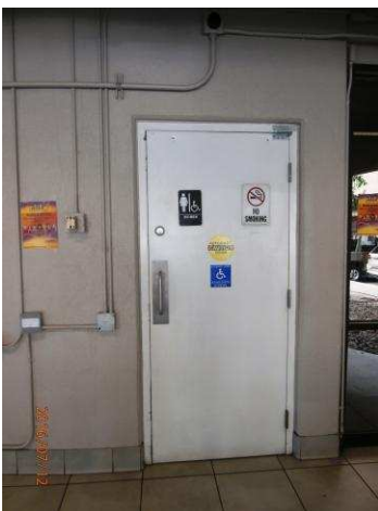
Image of noncompliant restroom signage
