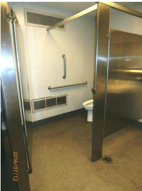
Image of narrow toilet stall
