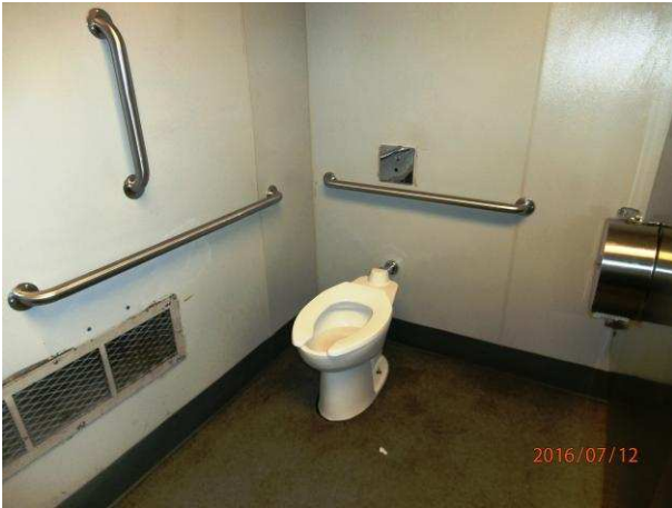
Image of toilet paper installed too far from toilet
