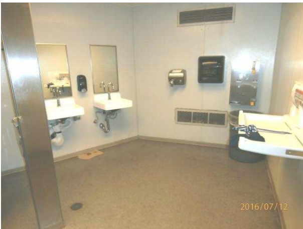
Image of noncompliant diaper changing station
