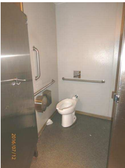
Image of narrow toilet stall
