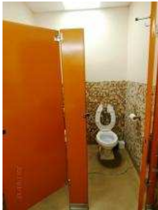
Finding 184833 Additional Photo
