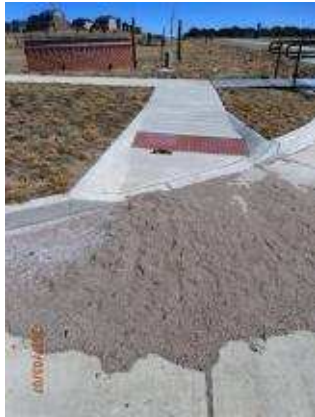
Finding 184965 Additional Photo
