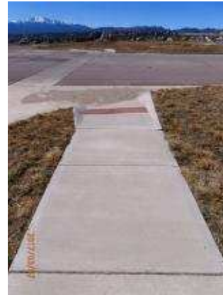
Finding 184965 Additional Photo
