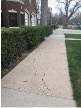
Finding 184223 Additional Photo
