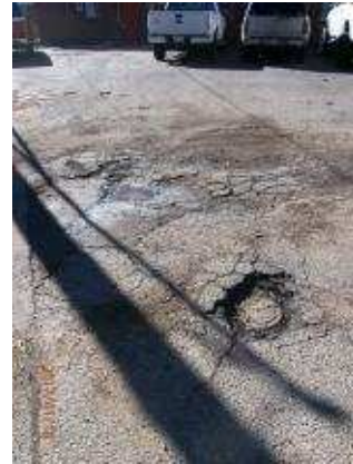
Finding 184231 Additional Photo
