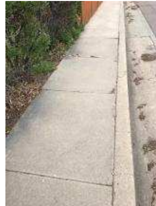
Finding 184233 Additional Photo
