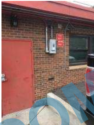
Finding 184231 Additional Photo
