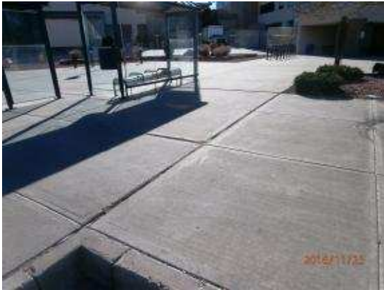
Additional image of gaps and vertical displacement
