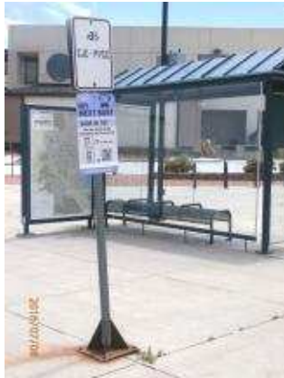
Additional image of displacement at bus stop
