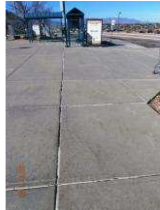
Additional image of gaps in sidewalk
