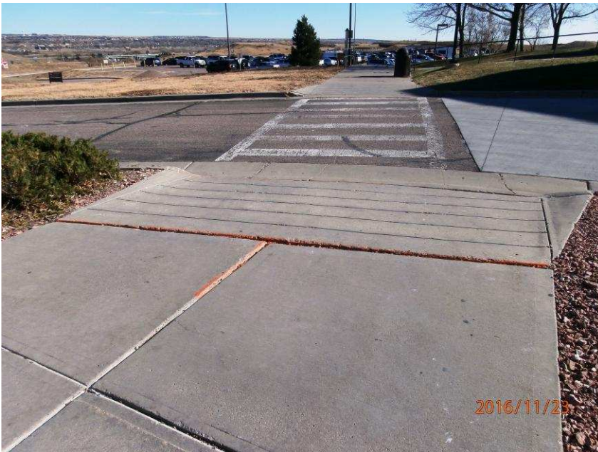
Image of noncompliant curb ramp
