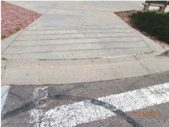
Additional image of noncompliant curb ramp
