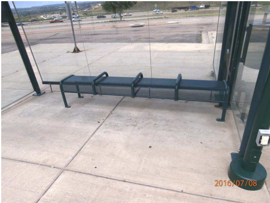
Image of vertical displacement at bus stop
