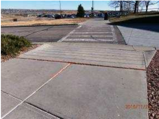
Additional image of gaps in sidewalk
