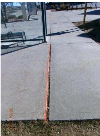
Image of sidewalk with excessive slopes
