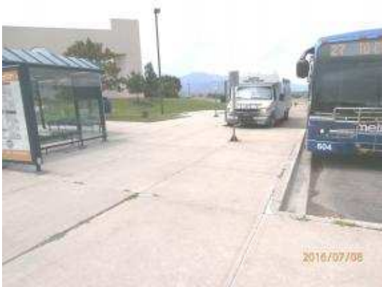
Additional image of gaps and vertical displacement
