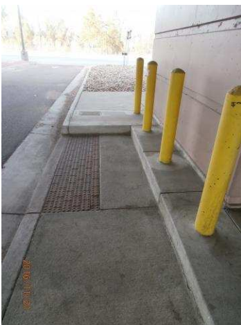
Image of curb ramp without fall protection
