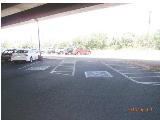
Image of accessible parking without signage
