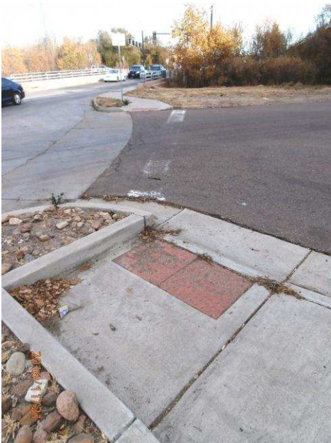
Image of noncompliant curb ramp
