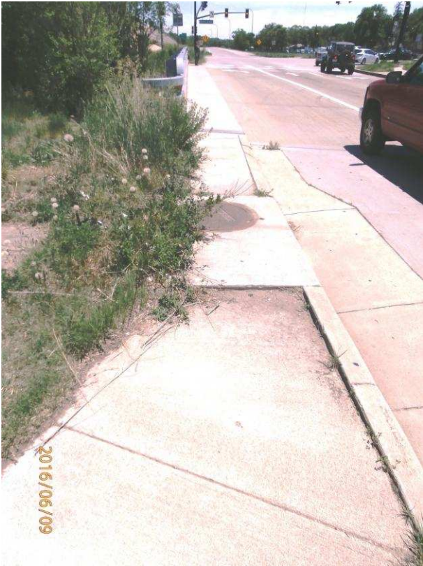
Image of vertical displacement at storm inlet
