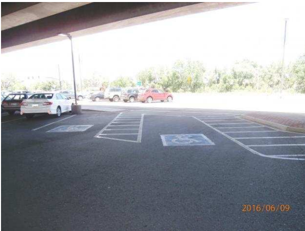
Image of lack of van accessible parking space
