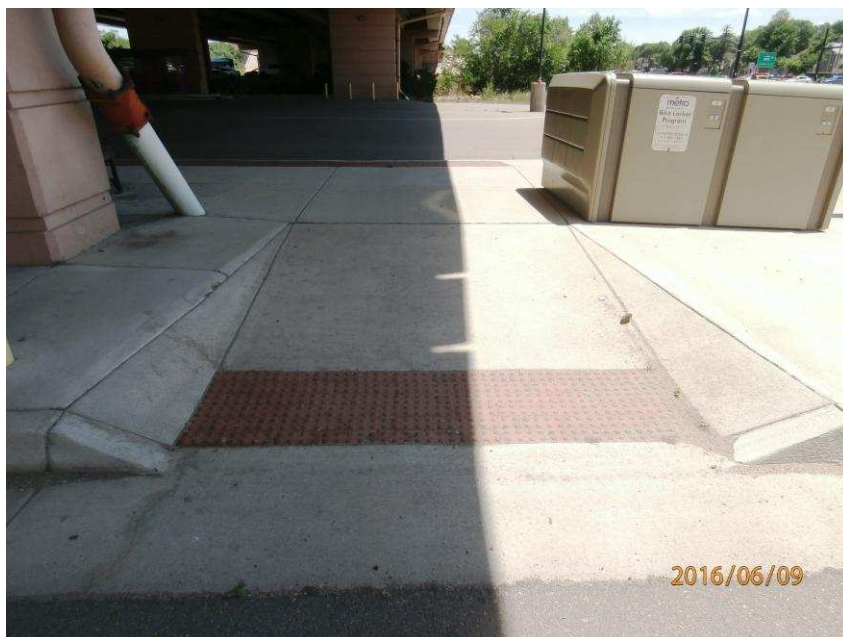
Image of noncompliant curb ramp
