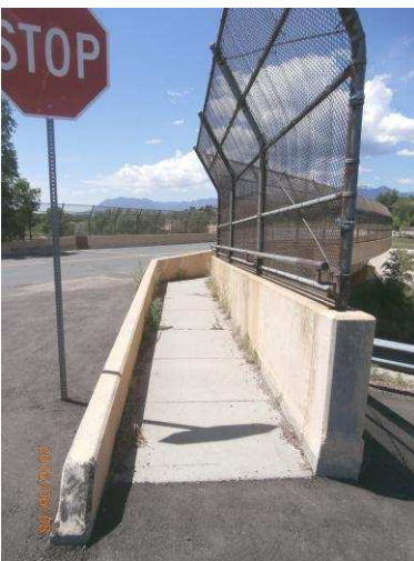
Image of sidewalk with vertical displacement
