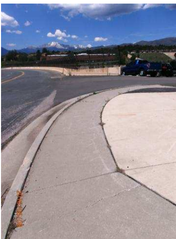
Image of sidewalk with excessive cross slopes
