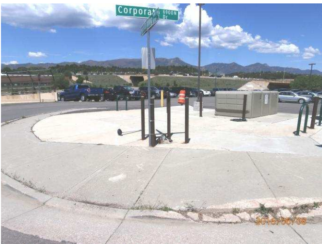
Image of noncompliant curb ramp
