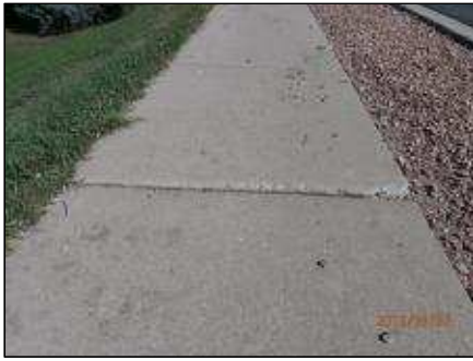
Vertical displacement in the sidewalk
