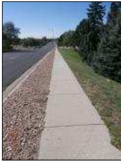
Sidewalk with excessive cross slope
