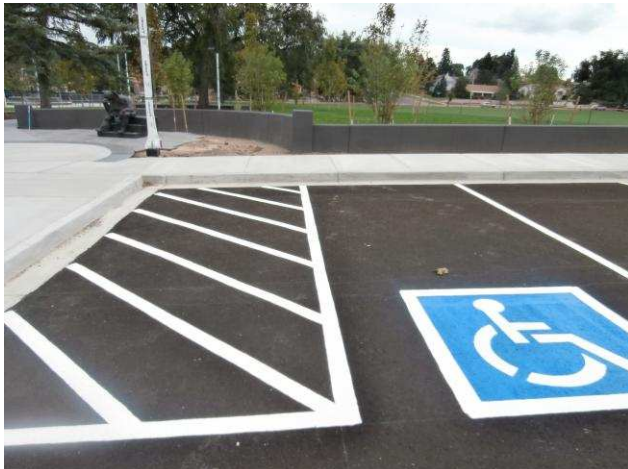
Image of access aisle with excessive cross slope
