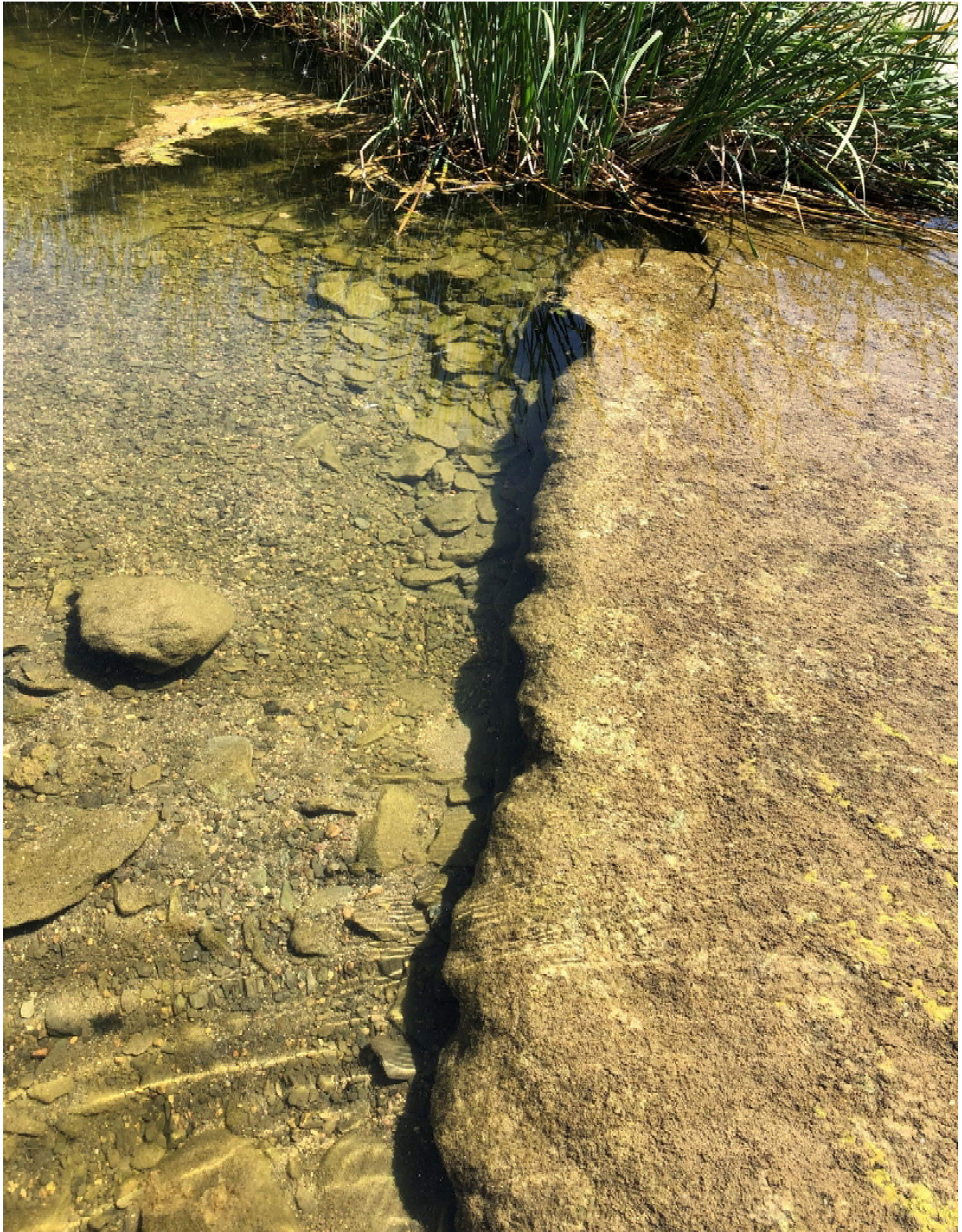
PHOTO AREA 1 - EROSION AND UNDERCUTTING AT HEADWALL/CREST - LOOKING EAST
