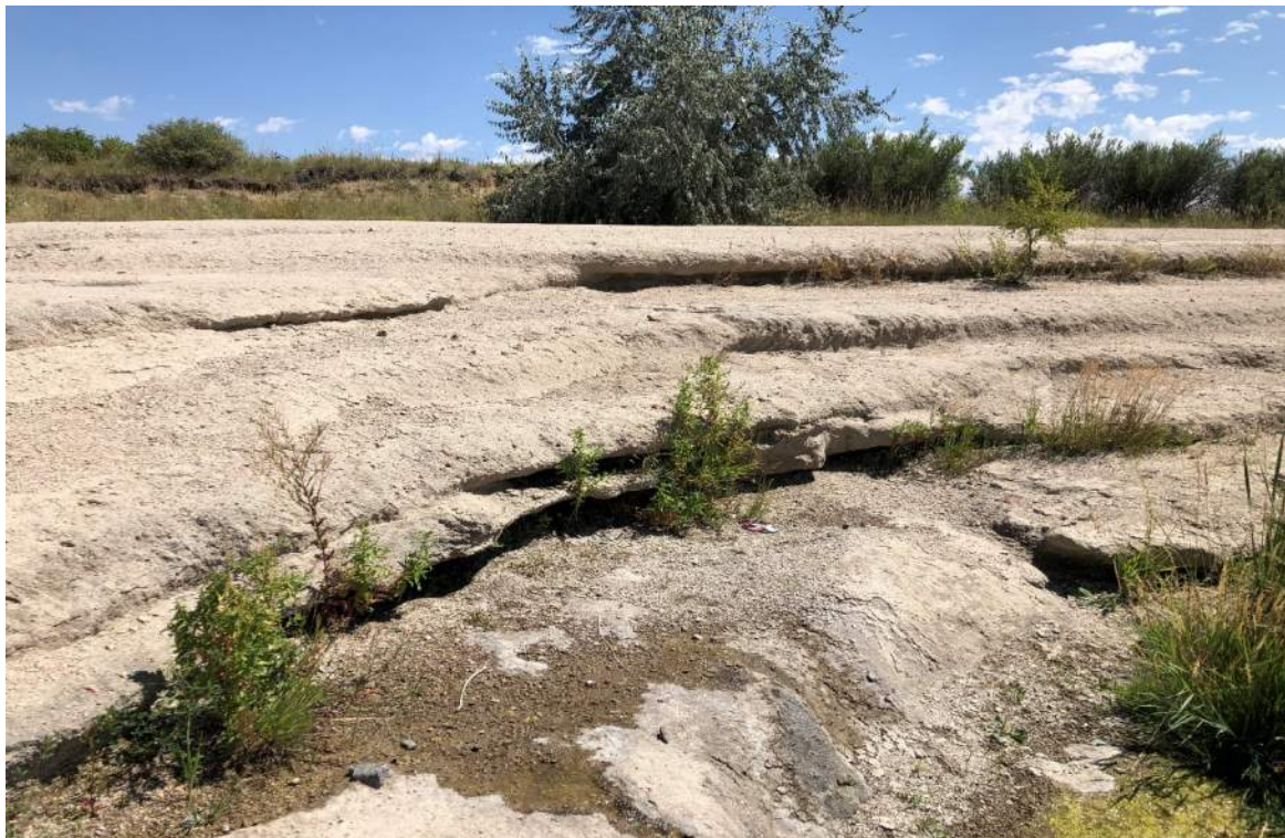
PHOTO AREA 3 - UNDERCUTTING OF EAST SIDEWALL - LOOKING EAST
