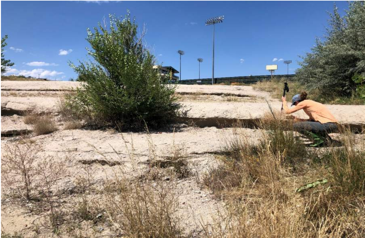
PHOTO AREA 2 - UNDERCUTTING OF WEST SIDE WALL - LOOKING NORTHWEST
