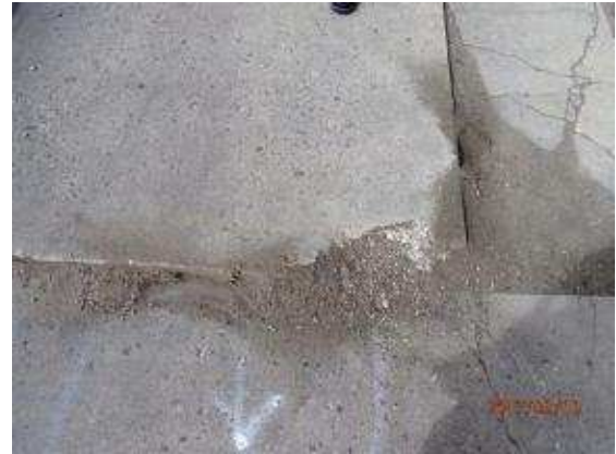
Finding 184777 Additional Photo
