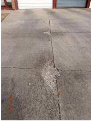
Finding 184779 Additional Photo
