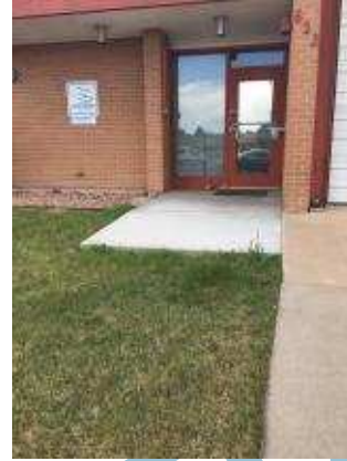
Finding 184782 Additional Photo
