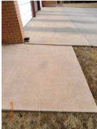
Finding 184781 Additional Photo
