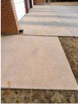
Finding 184782 Additional Photo
